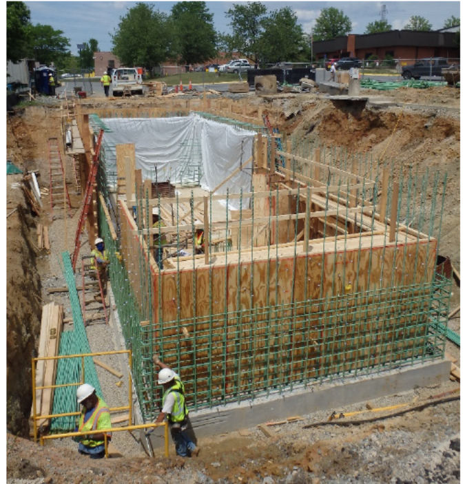
GKY's work for Fairfax County includes design and construction administration for retrofit structures such as this sand filter and a nearby bioretention BMP at the Newington Solid Waste Facility.
