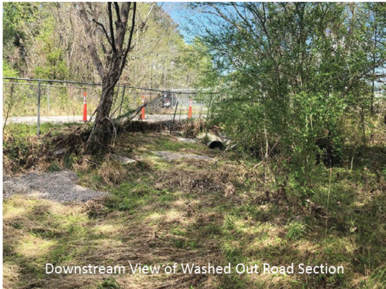
Washed Out Road Section to Sludge Fields
