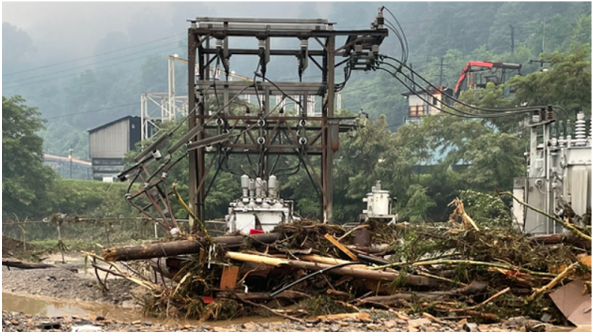
Figure 6-23: Flood damage at Appalachian Power's Dismal River Substation, 2022 39
