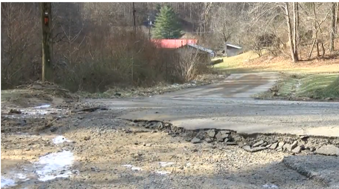
Figure 6-14: 2019 mine blowout damage near Hurley, VA
