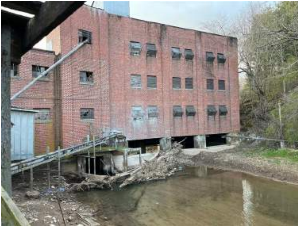
Figure 32: Abandoned Farm Bureau Building capturing debris.
