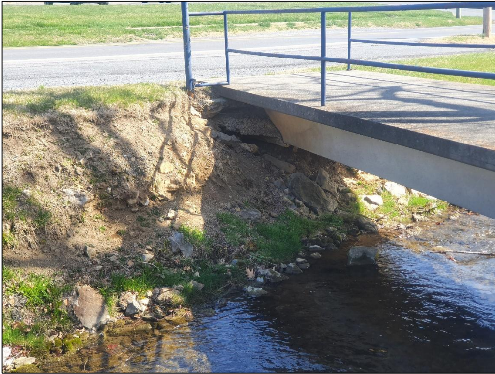
Photo 3. Bank Erosion under Pedestrian Bridge spanning Abrams Creek
