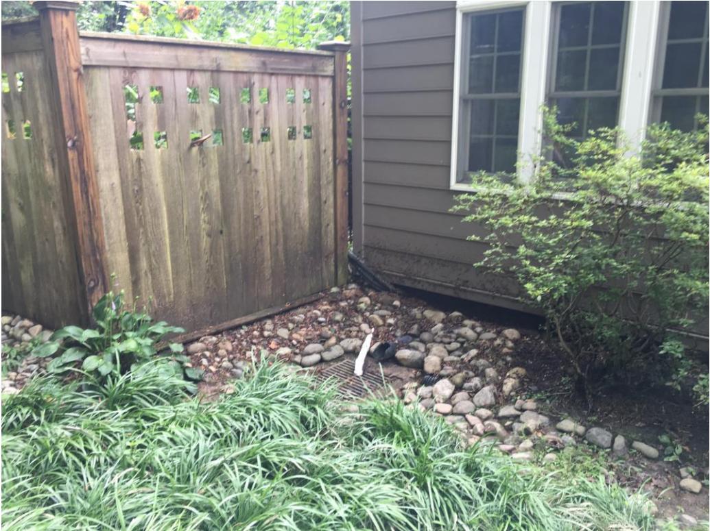
Figure 1: Post Flood Pictures
