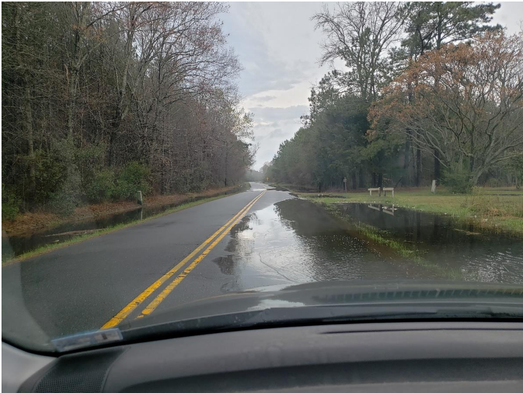
Photo 2: Flooding of ditches and road on Church Neck Road, the only access to communities extending down Church Neck, due to rainfall and inadequate drainage.
