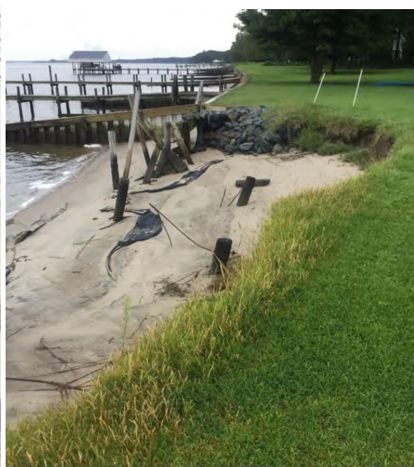
Photo failing bulkhead, rip rap, and eroding land.
