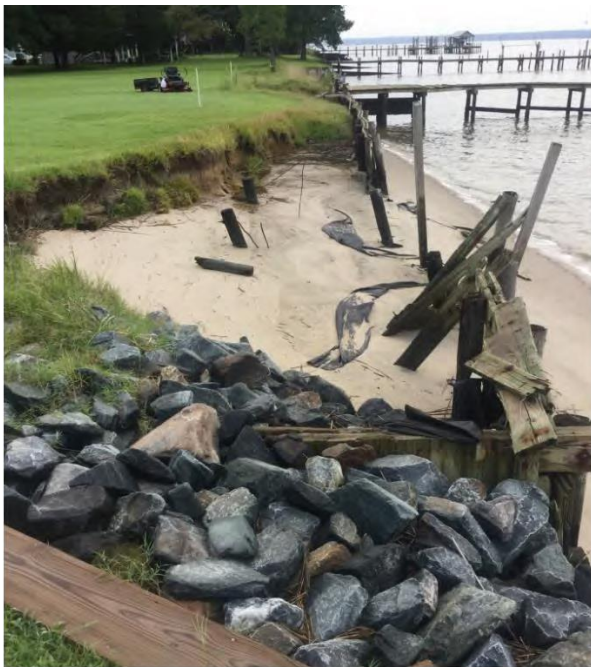
Rip rap placed behind failing bulkhead and attempting to hold the land in place.
