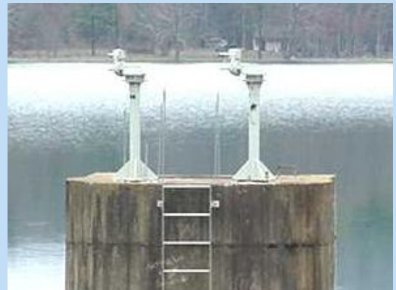
Typical Gate Operators 44
