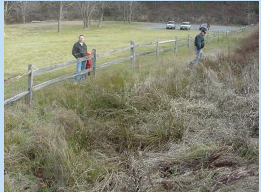
Seepage and/or Wet Spots on the Toe
