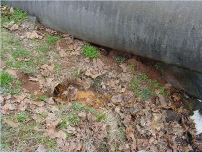
Toe Drain Blocked – Not flowing freely
