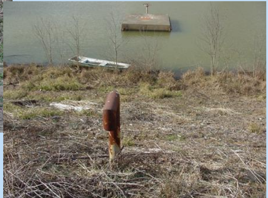
Air Vent Pipe
