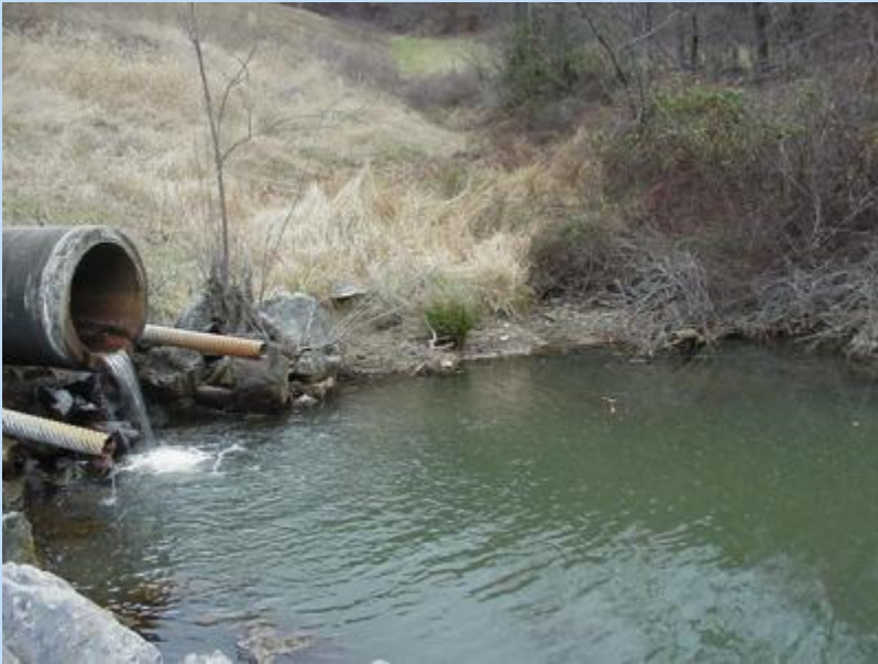
Rip Rap Missing Or Displaced
