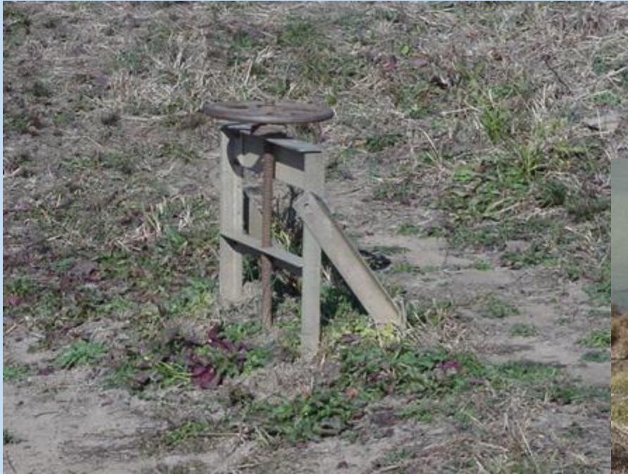
Potential Piping Sources Sluice Gate to Mill
