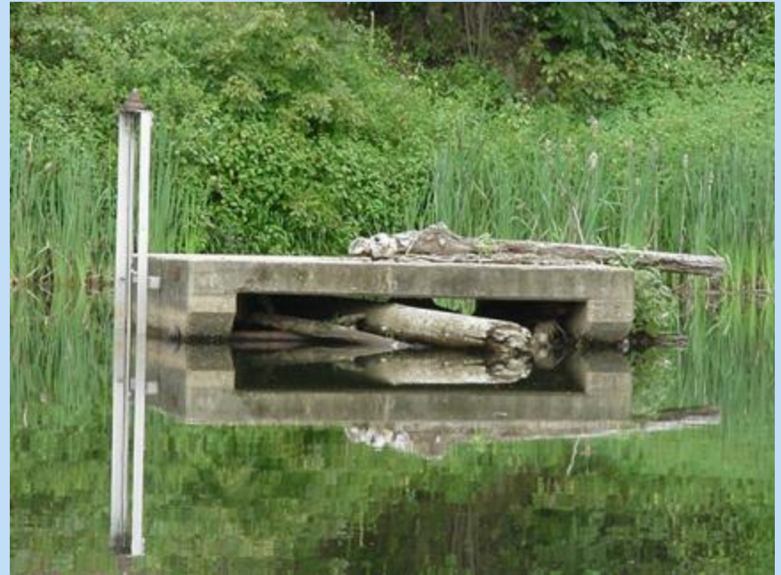
Tower with Debris on Top & In Riser Tower Weir Opening
